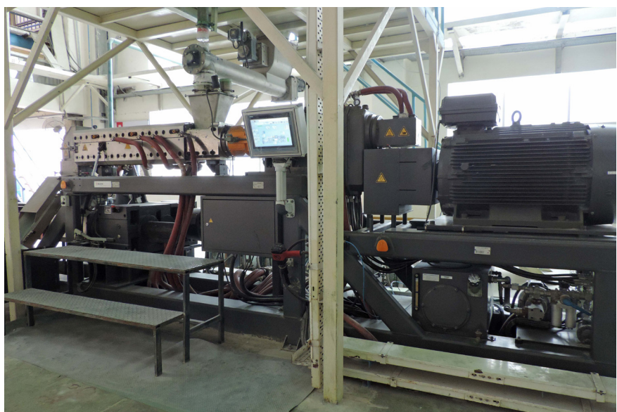
BUSS Kneader plant
